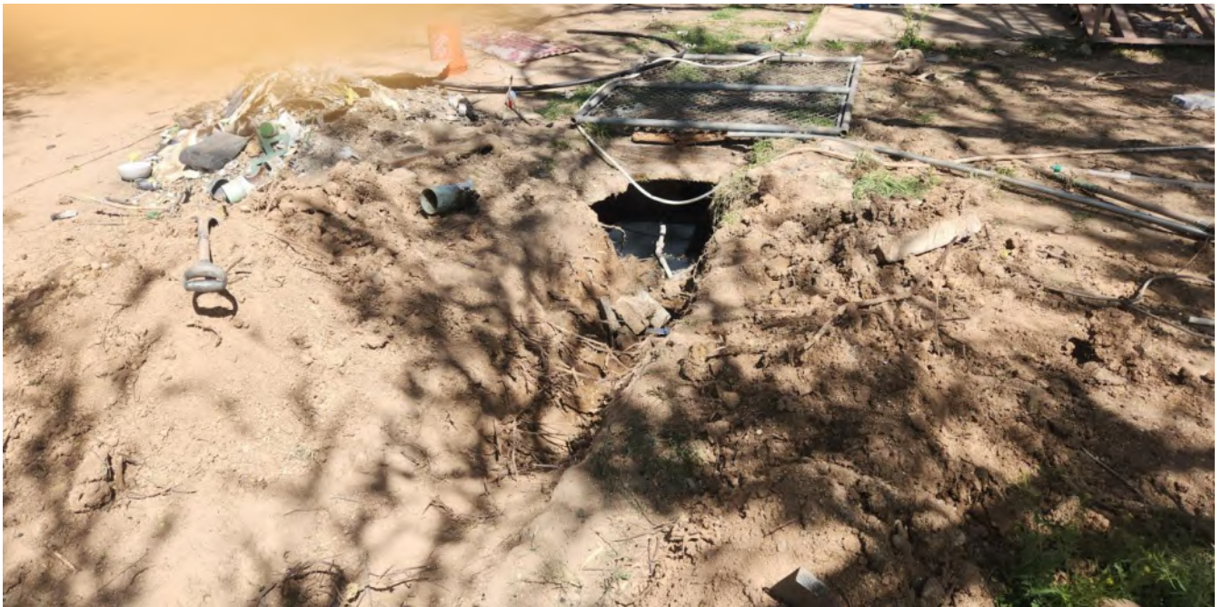
SEPTIC SYSTEM DAMAGED
