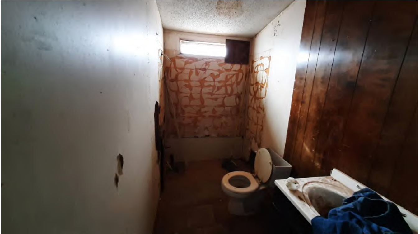
BATHROOM PLUMBING DAMAGED.
