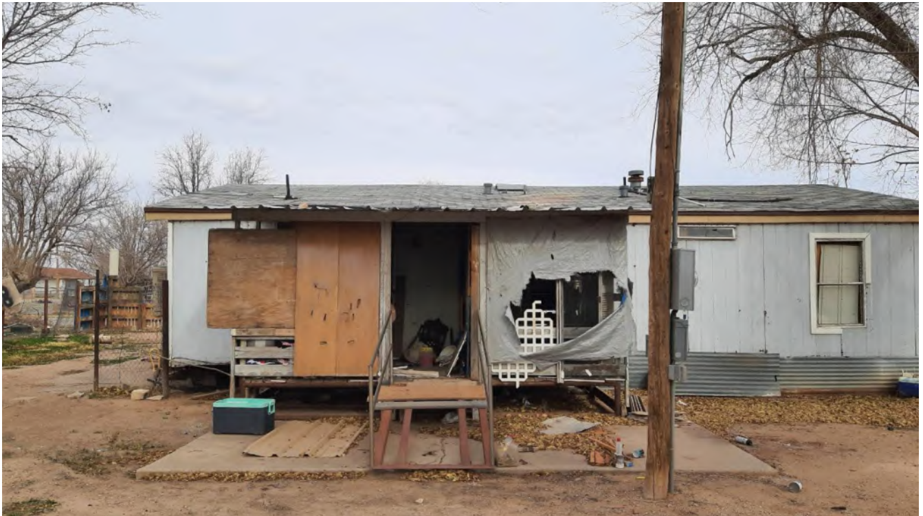
BACK SIDE OF THE STRUCTURE. ROOF FAILING.
