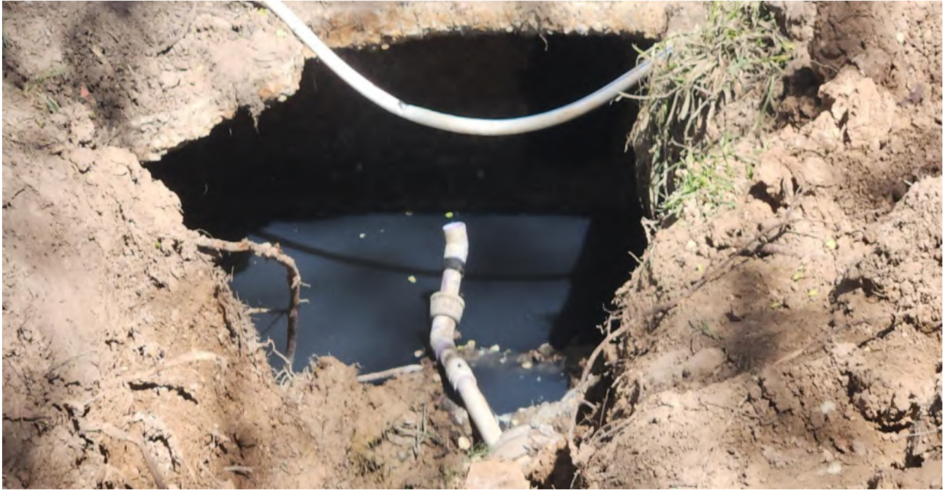
SEPTIC SYSTEM DAMAGED
