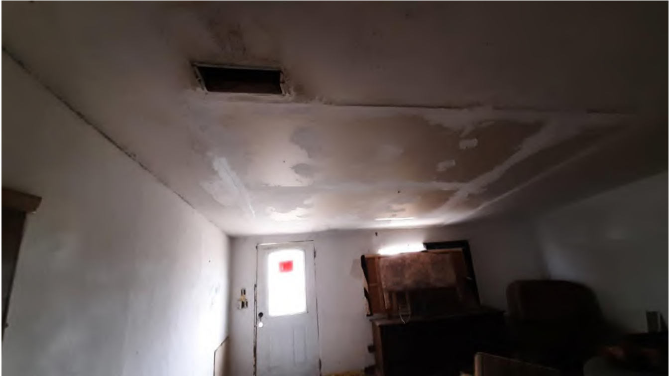
FAILING CEILING PATCH
