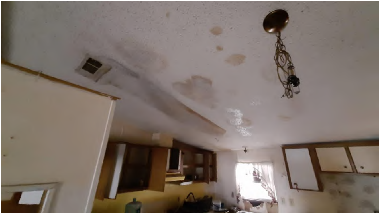
MOLD AND ROTTEN CEILING
