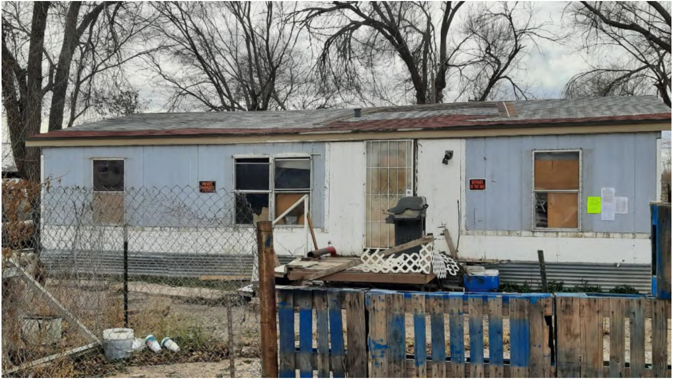
FRONT SIDE OF THE STRUCTURE. ROOF FAILING
