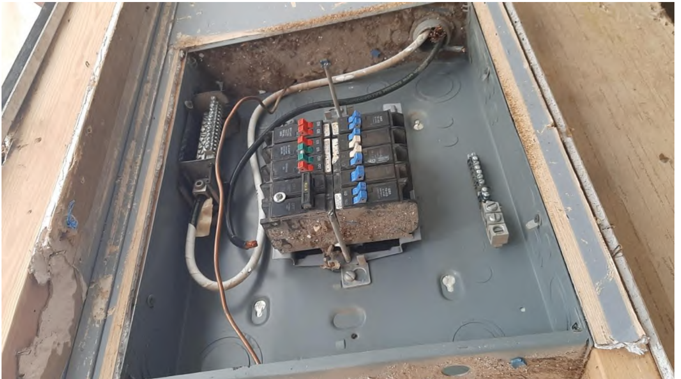
ELECTRICAL PANEL DAMAGED.
