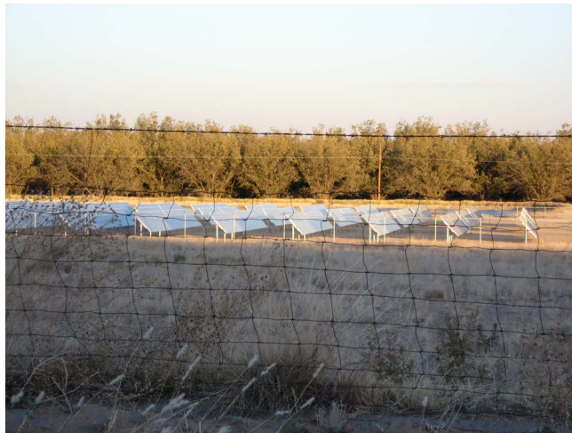
Relatively new solar project located in the ETZ
